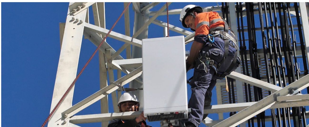
Installation of Ericsson's 5G radio masts at Telstra's innovation Centre in Australia. Source: Ericsson
