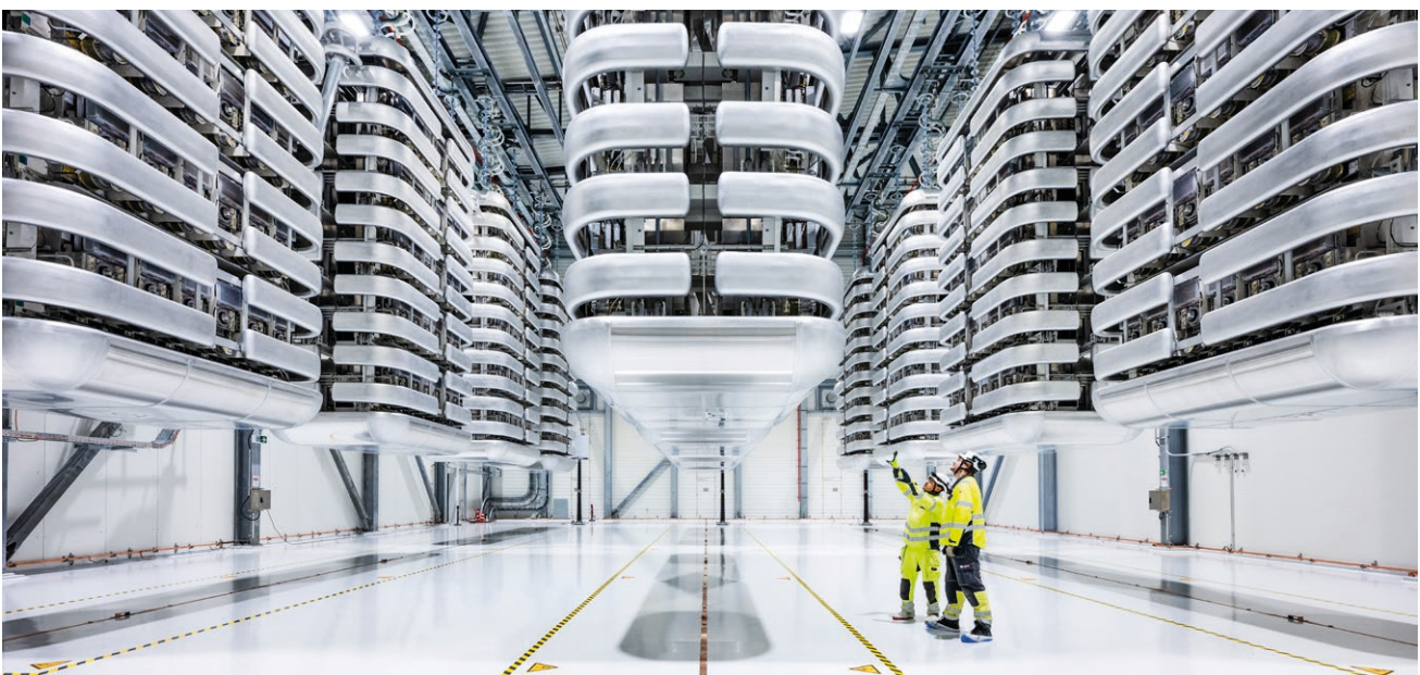
The high-voltage direct current (HVDC) conversion station in Emden, Germany, transmits electricity for up to one million households from offshore wind power in the North Sea. Source: Hitachi Energy, Ludvika.
